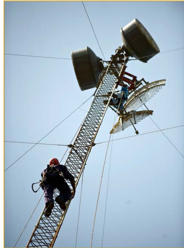
Electrical technicians of the Communications Information Technology Section of the United Nations Mission in Liberia works on the radio tower in the Bomi County. (UN Photo #325801, Christopher Herwig, February 2009)
